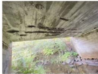
Soffit Excessive Severe Delamination & Exposed Rebars
