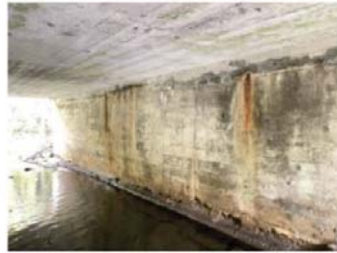
Wet Rusted Med to Severe Cracks on East Wall
