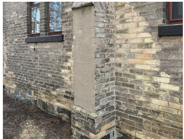
Fig. 5.17. West elevation, buttress with parging and localized deterioration at lower portion
