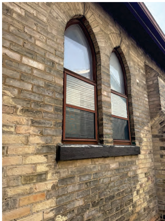
Masonry cracking at the pointed window arch
