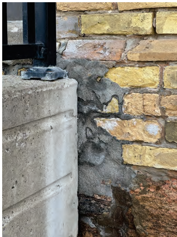
Cementitious repair and deterioration at junction with brick masonry
