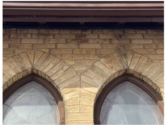
Fig. 5.15. Masonry cracking at the pointed window arch
