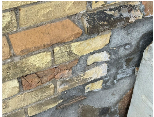
Fig. 5.16. Localized brick spalling and mortar deterioration at base
