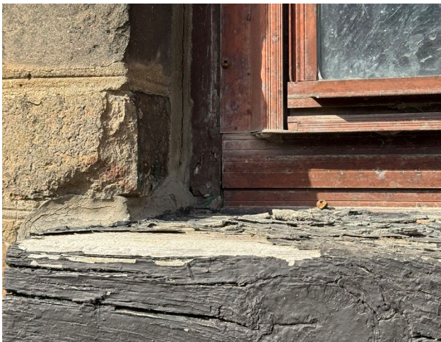
Fig. 5.13. Window sill and jamb showing weathering, and localized deterioration
