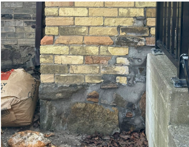
Fig. 5.8. Foundation and lower wall showing brick deterioration, and incompatible repair
