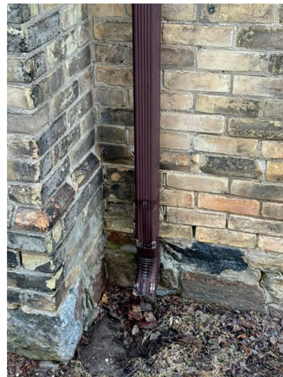
Downspout discharge at foundation with localized masonry deterioration
