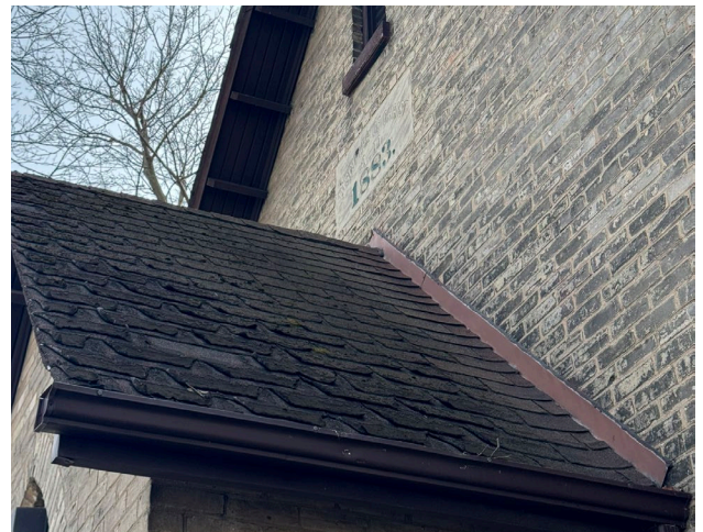
Fig. 5.5. Front entrance, asphalt shingle roof at the front entrance in poor condition and evidence of biological growth
