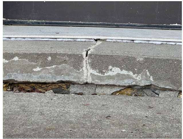
Fig. 5.4. Front entrance, cracking and deterioration at base of entrance
