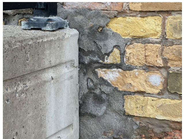
Fig. 5.6. Front entrance, parging and deterioration at junction with brick masonry
