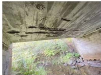
Soffit Excessive Severe Delamination & Exposed Rebars
