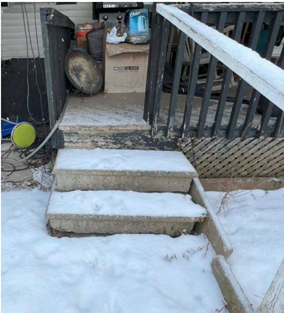
Painted wood on the rear porch in fair to poor condition (ERA, 2025).
