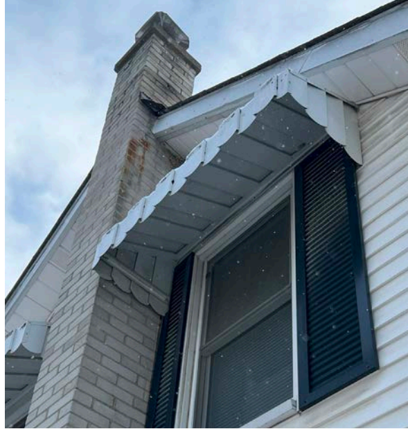
Modern vinyl windows and metal awnings and shutters at the north (side) elevation in fair condition. Modern brick chimney in fair condition with minor deterioration towards the top (ERA, 2025).
