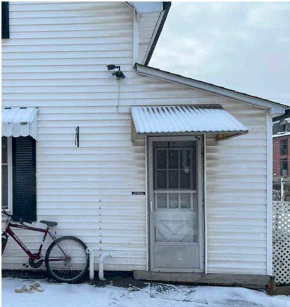
Vinyl siding at the north (side) elevation in fair condition, with some soiling and organic growth visible (ERA, 2025).
