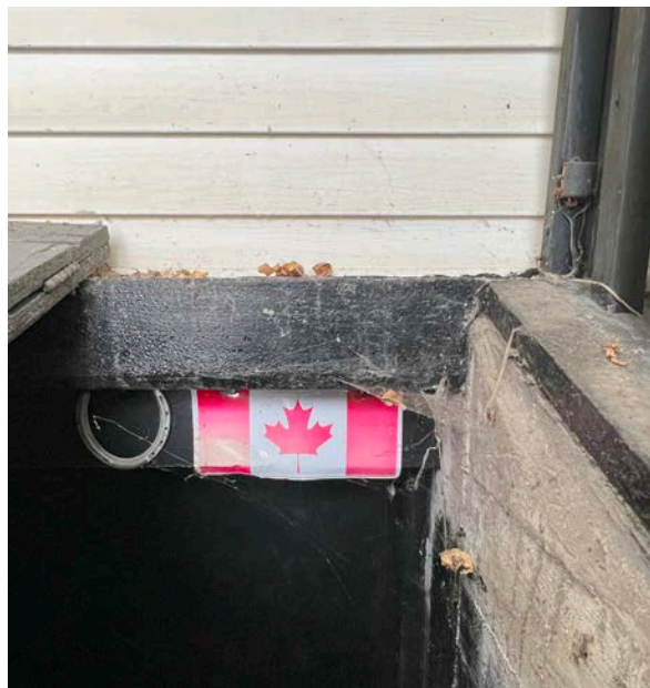
Timber lintel over the basement door at the rear (west) elevation provides evidence of an older structure (ERA, 2025).
