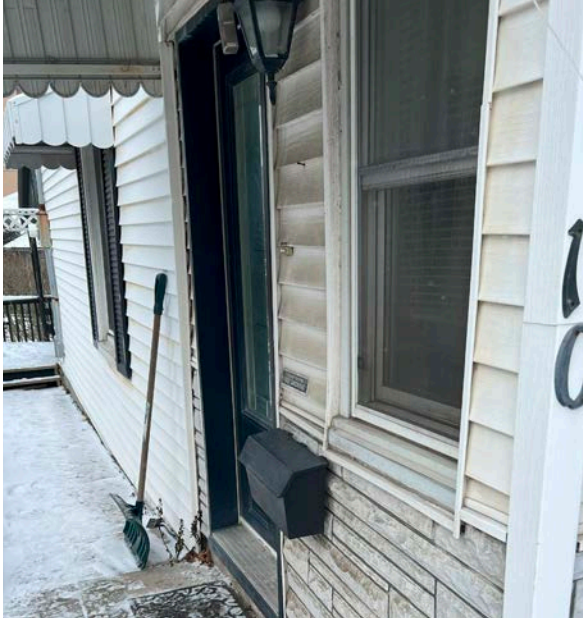
Modern vinyl window inserts, contemporary door, and metal awnings in fair condition (ERA, 2025).
