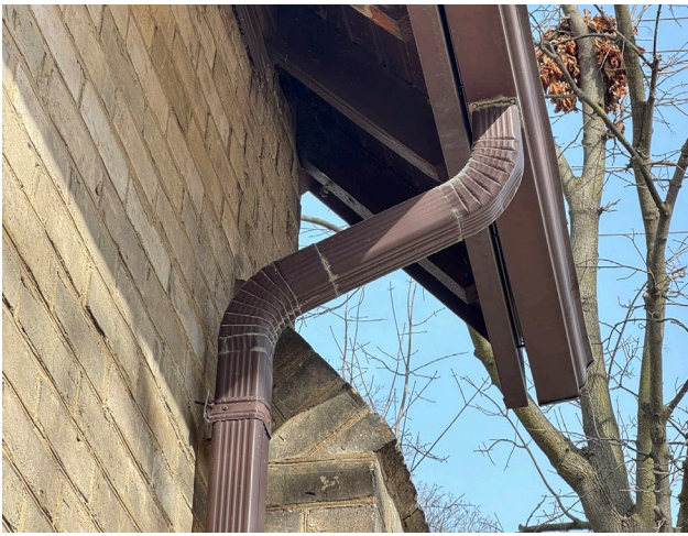
Fig. 5.12. Eaves, soffit, and downspout showing existing rainwater management and roof edge
