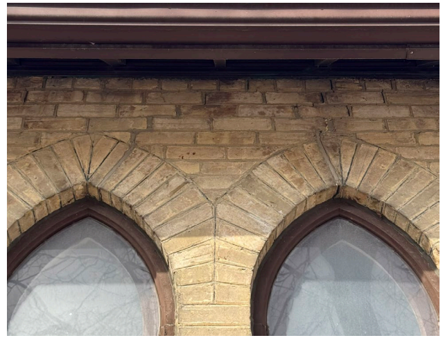
Fig. 5.15. Masonry cracking at the pointed window arch
