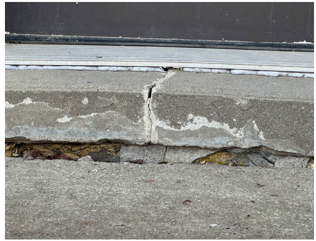
Fig. 5.4. Front entrance, cracking and deterioration at base of entrance
