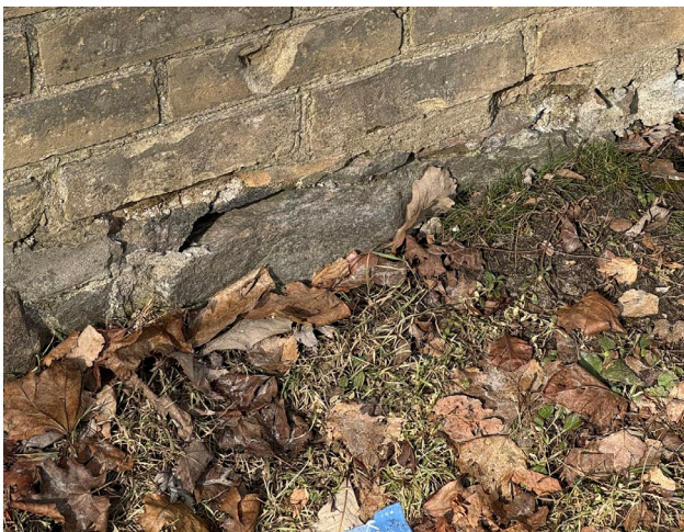
Fig. 5.11. Mortar loss and cracking at the foundation stone, brick weathering
