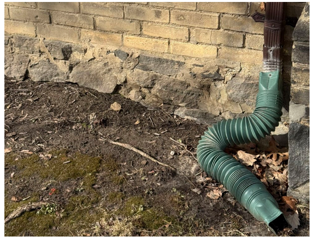
Fig. 5.9. Northeast corner, condition of lower buff brick wall and downspout area
