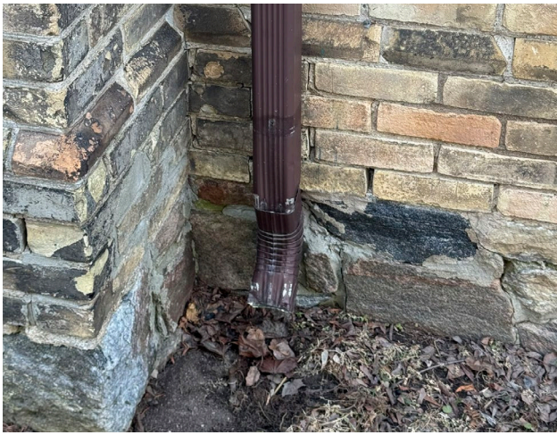
Fig. 5.7. Northwest corner, downspout discharge at foundation with localized masonry deterioration
