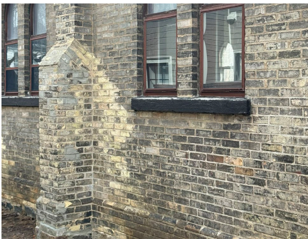
Fig. 5.3. West elevation, typical butters condition and localized masonry weathering
