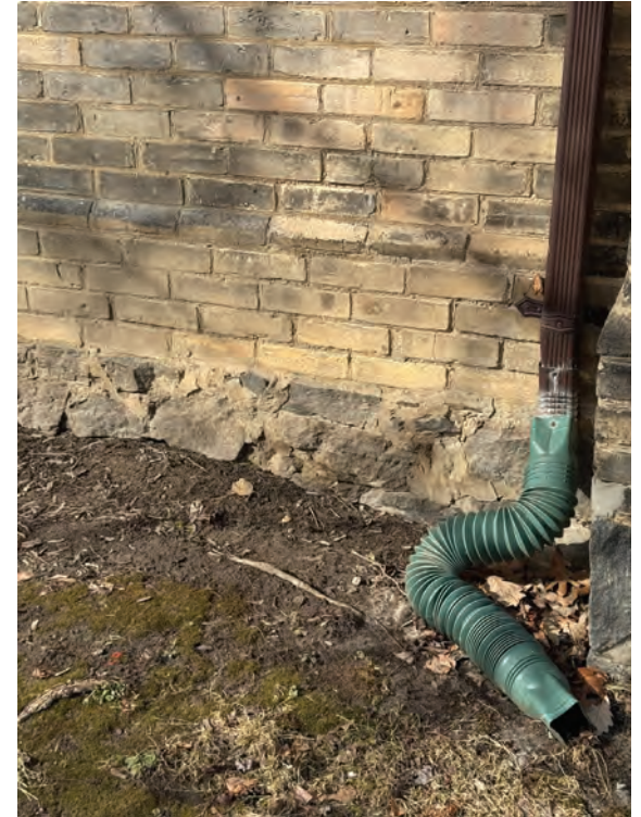
Condition of lower buff brick wall and downspout area
