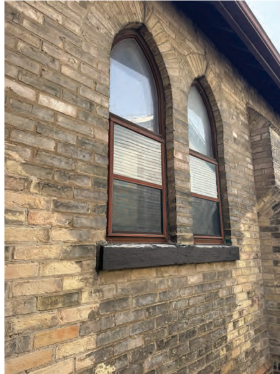
Masonry cracking at the pointed window arch
