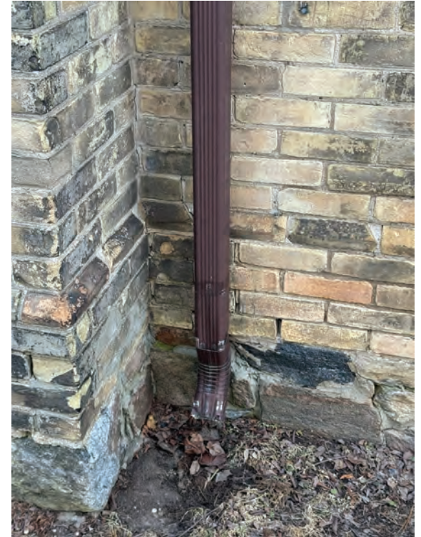
Downspout discharge at foundation with localized masonry deterioration
